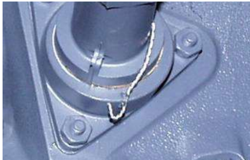
Figure 2 Safety Wire on the Oil Level Gage
